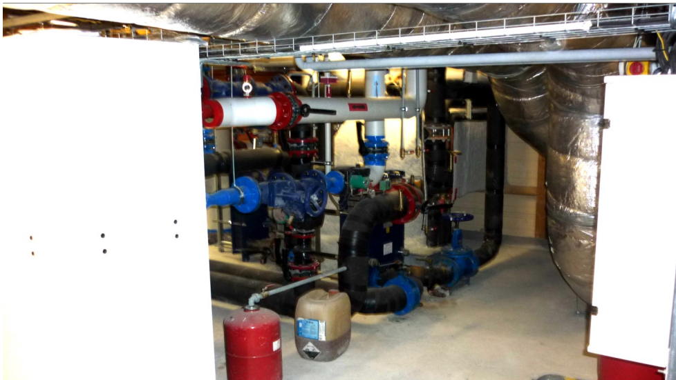
Local technique chauffage ventilation
